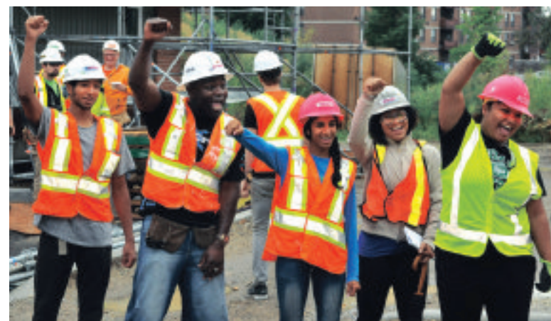
Three cheers for progress! One Team One Voice high school all-star team members “getting their build on”.
