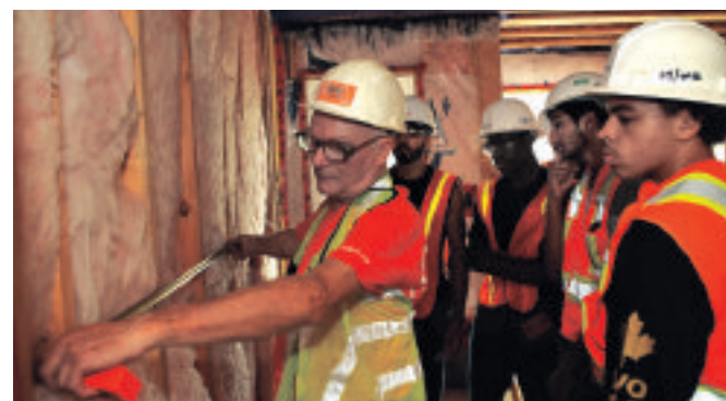
Showing the One Team One Voice all-stars how to install drywall is crew leader Bob Rutledge.
